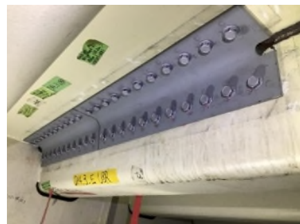
写真-2 TRS工法を用いた当て板状況 Photo 2 Installation of TRS method
