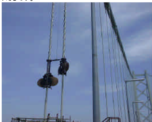
新開発の巻付機で格点毎に2本同時に施工 Newly developed robot winds two helical ropes simultaneously around a pair of hangers
