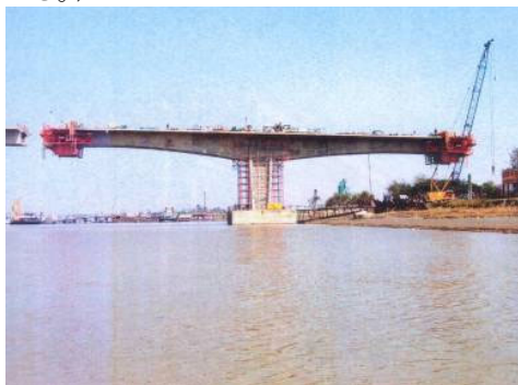
写真-4 本橋7Pの施工状況(1月末) Photo.4 View of Main Bridge at MP7 (End of Jan.)
