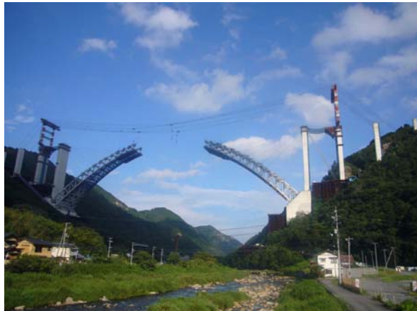
写真-4 空港大橋の架設状況全景 (Photo.4 Construction status of Airport Bridge)
