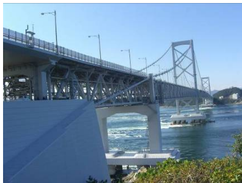
写真-1 耐震補強中の大鳴門橋 (Photo.1 Seismic retrofit work underway on Onnaruto Bridge)
