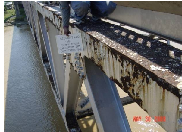
写真-4 補剛桁上弦材の錆 (Photo.4 Corrosion on upper chord of girder)
