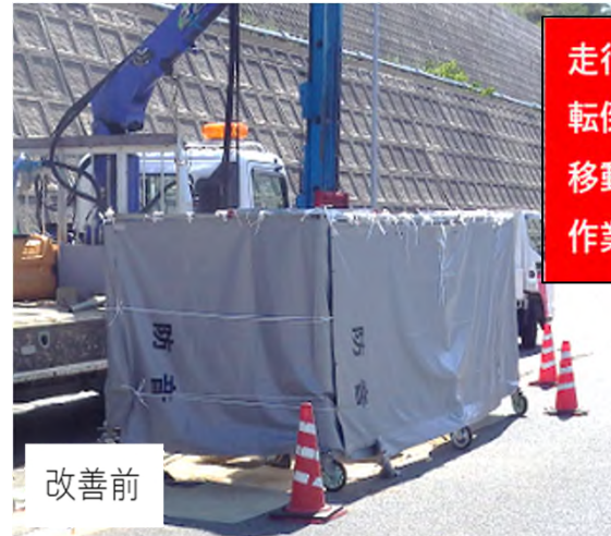
[改善前] R1発注工事 H=1.5m, L=4.0m, W=1.8m
