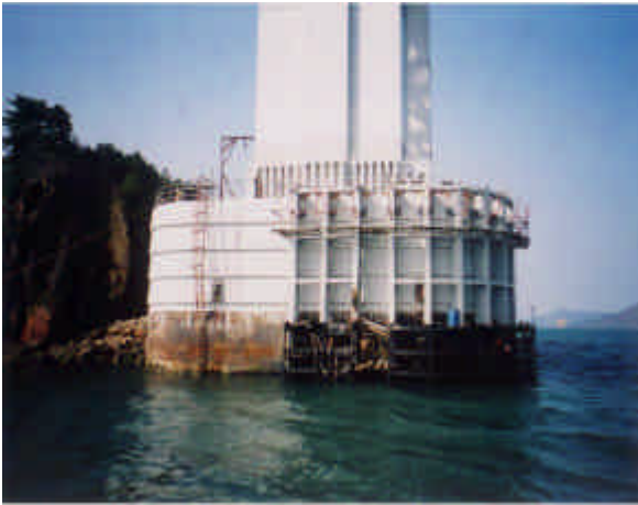
緩衝工損傷状況 (Damage of the Buffer System)
