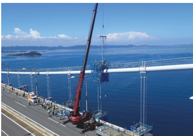
写真-1 旧ロープの撤去状況 Photo 1 Situation of the Removal of Old Suspender Ropes
