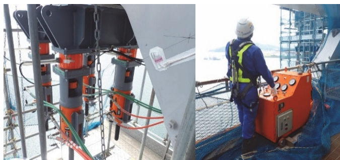
写真-2 新ロープ設置時の張力調整状況 Photo 2 Tension Adjustment during the Installation of new suspender ropes
