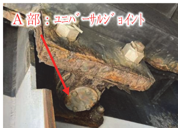
写真-1 腐食状況 Photo 1 Corrosion Status of the Joints
