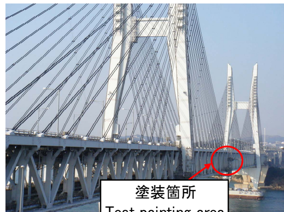
写真-1 実橋試験塗装(櫃石島橋) (Photo.1 On site test painting at Hitsuishijima Bridge)
