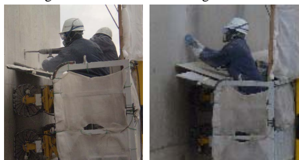
写真-3 ドリル穿孔、壁面補修の状況 (Photo.3 Drilling and repair work of concrete wall using vacuum wheeled gondola)
