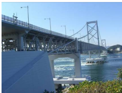
写真-1 耐震補強中の大鳴門橋 (Photo.1 Seismic retrofit work underway on Onnaruto Bridge)
