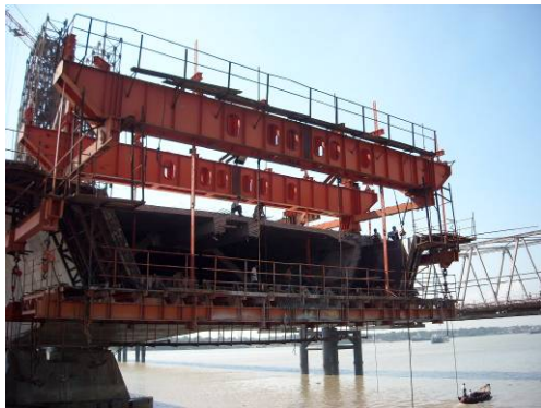
写真-3 PC 桁の張出架設(後方のトラス橋は既存のシャー・アマナト橋) (Photo.3 Cantilever erection of PC girder (the existing truss bridge in the back))
