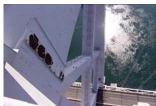
写真-1 鋼製カバーの腐食 (Photo.1 Corrosion on steel cover)
