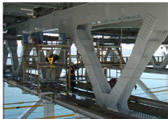
写真-2 小組トラスのスライド足場 (JR委託) Photo-2 Sliding Scaffolding for small truss members above train lines. (by JR Shikoku)
