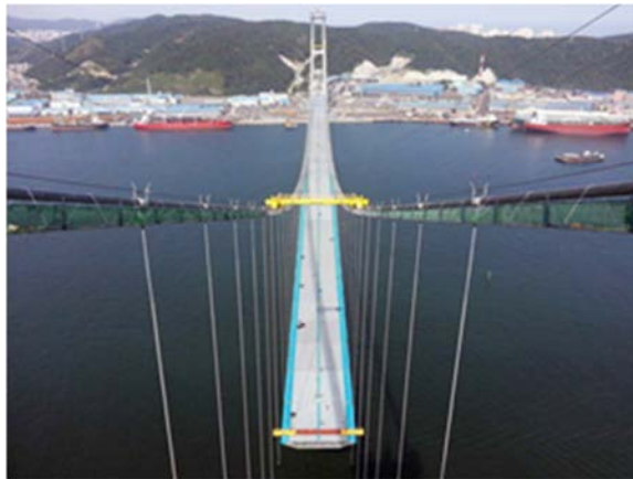
写真-6 補剛桁架設中の塔頂からの全景 Photo.6 View from tower top during erection of girder
