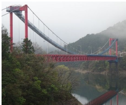
写真-3 上吉野川橋(調査吊足場) Photo. 3 Kamiyoshino-gawa Bridge (Cat-walk for investigation work)
