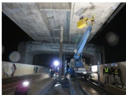
写真-2 軌陸車による夜間点検・補修 Photo-2 Night-time inspection and repair with road-rail vehicle
