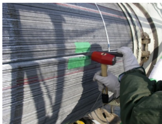
写真-1 くさび打ちによる内部鋼線状況確認 Photo-1 Main cable internal inspection (cable wires were wedged)
