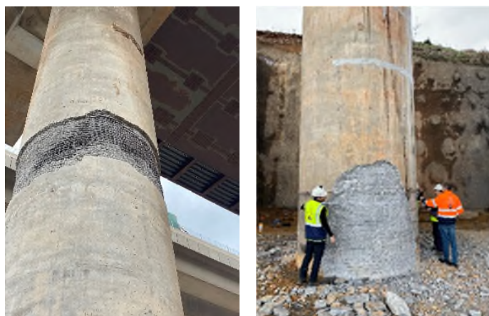
写真-5 橋脚の局部座屈 Photo 5 Pier damage due to local buckling
