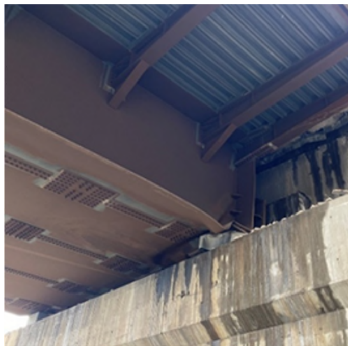
写真-6 箱桁端部の損傷 Photo 6 Box girder damage at bridge end.
