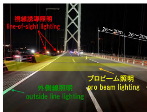
写真-2 橋梁用低位置道路照明(試験中) Photo 2 Low-position road lighting for bridges (under test)
