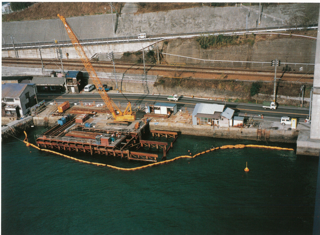
新尾道大橋 2P [棧橋設置工] New Onomichi Bridge 2P—Work pier installation
