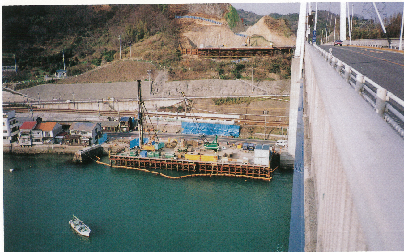
新尾道大橋 [尾道側下部工施工状況] Shin Onomichi Bridge - Sub structure Work on Onomichi side
