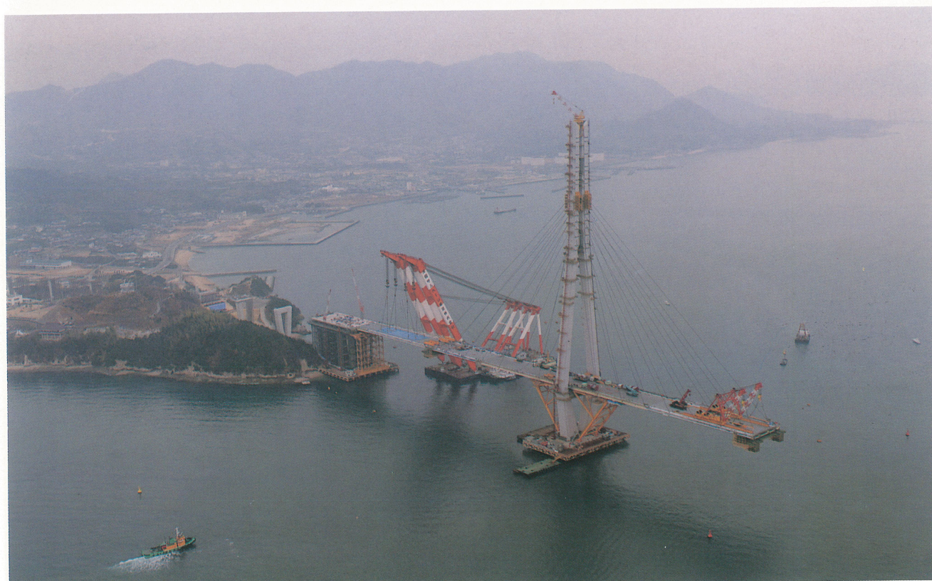
多々羅大橋 [3P側架設状況] Tataro Bridge - Erection Work on 3P side
