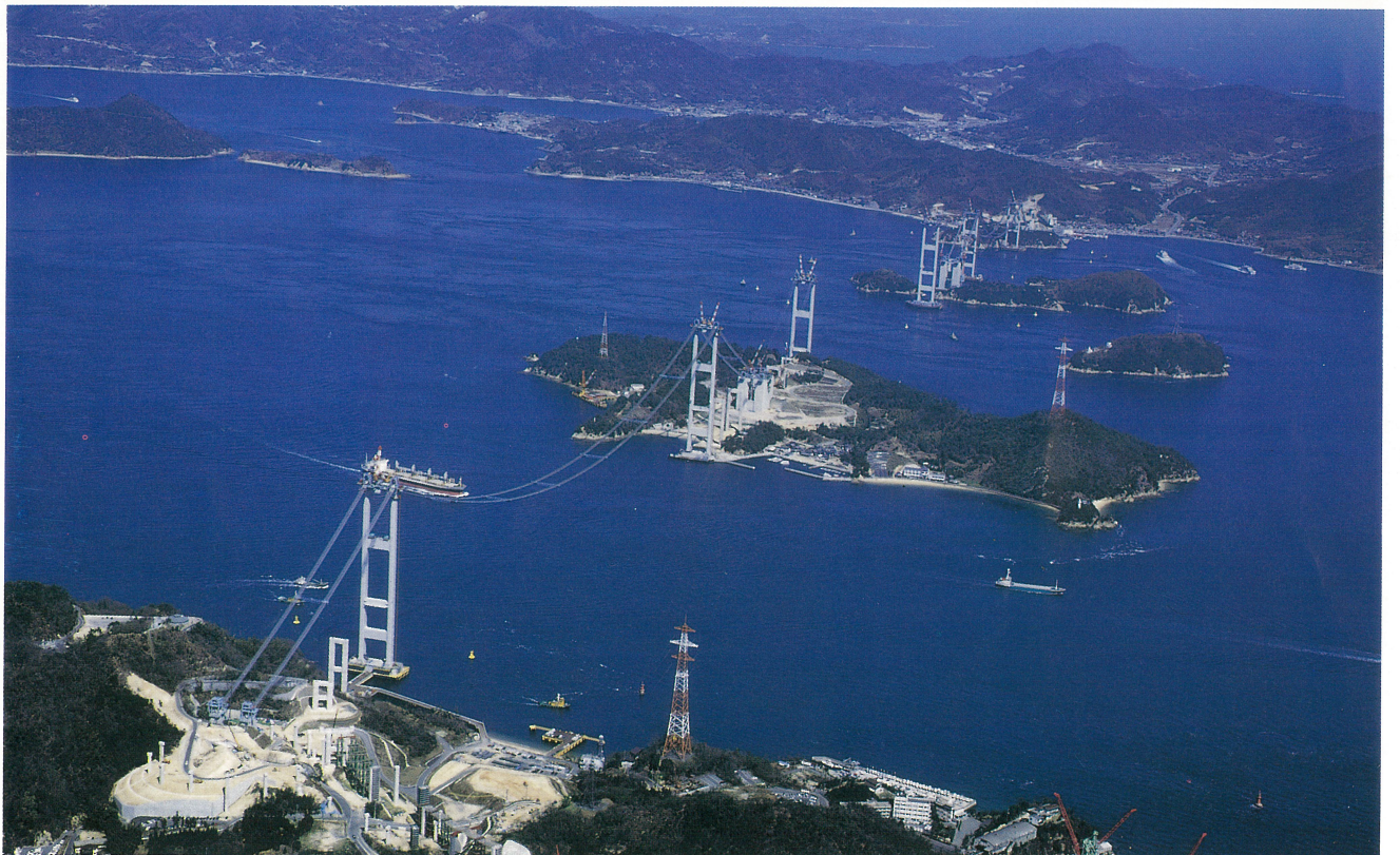
来島大橋全景 [今治上空より望む] Overview of Kurushima Bridge— from Imabari
