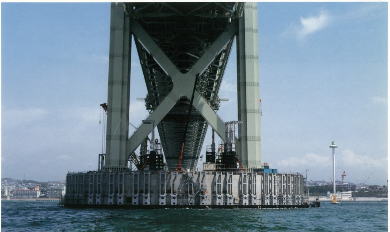
明石海峡大橋 2P 緩衝工工事 Akashi Kaikyo Bridge—works on buffer systems for the tower 2P
