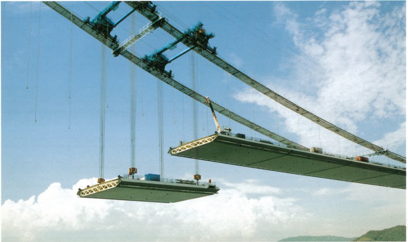
来島第一大橋 補剛桁架設状況 First Kurushima Bridge—erection of stiffening girder
