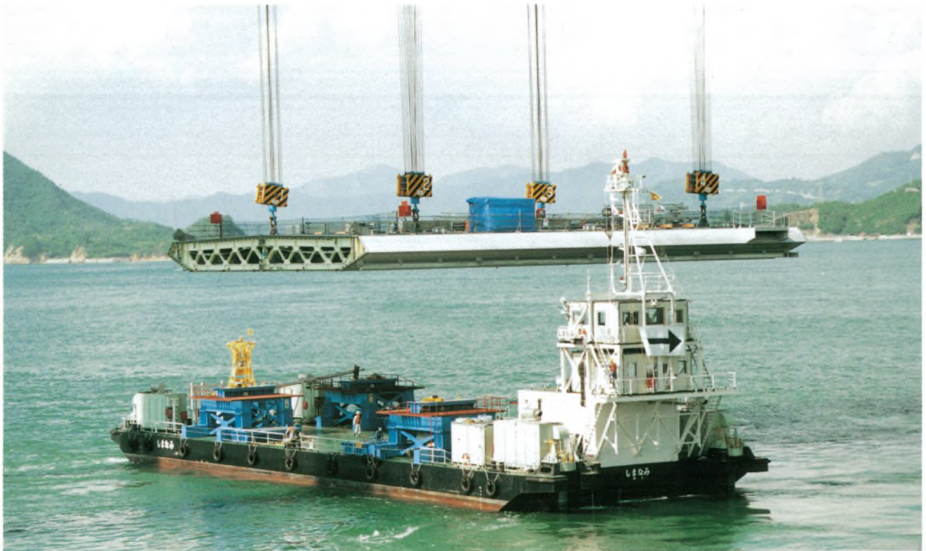
来島第一大橋 補剛桁架設状況 First Kurushima Bridge—erection of stiffening girder
