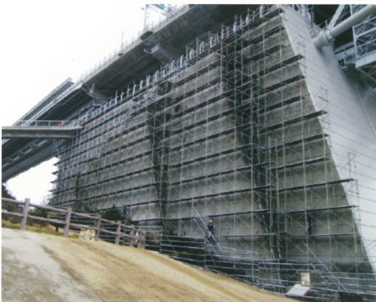
1A 全景 (瀬戸内海側の塗装足場) Overview of 1A (scaffolding on Setonaikai side)
