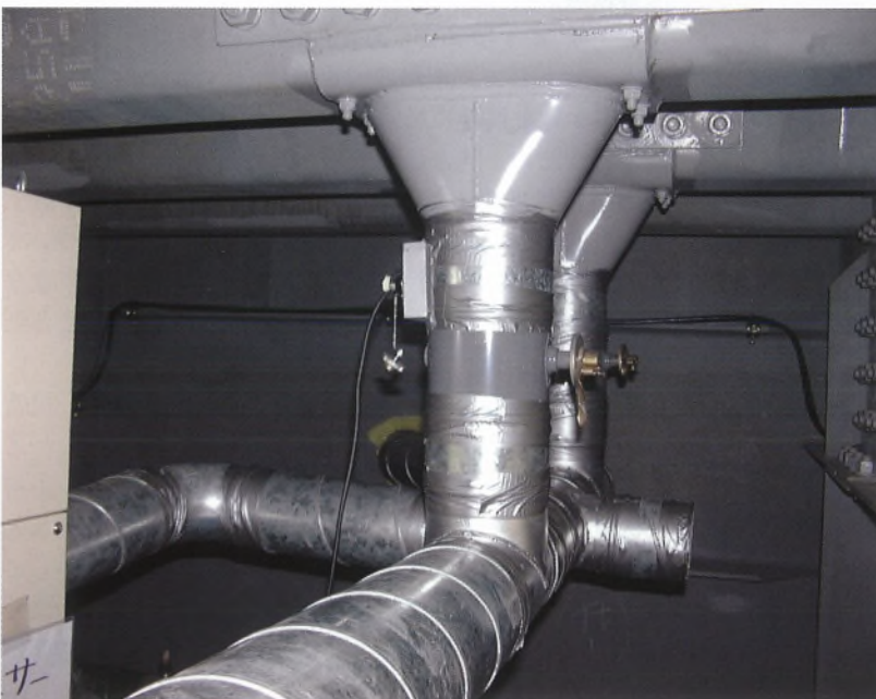
桁内機器設置状況 (手前側が除湿機、右奥がフィルタ) Installation of device in the deck (dehumidifier is on front side, filter on right-back)
