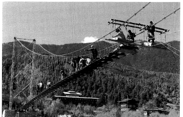
写真-5 吊橋架設状況 (写真提供 DOR) 少数の技術者、技能工の指導の下で村人が工事を進める Photo.5 Erection of a suspension bridge (Offered by DOR) Local people work under supervision by a few engineers and technicians
