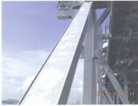
写真-3 上塗りと中間層剥離 photo.3 Peeling-off of top and middle coats
