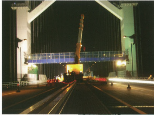
写真一1 主塔塗替塗装のための路面防護工夜間架設 Photo.1 Installation of Road Protection against falling object in night time
