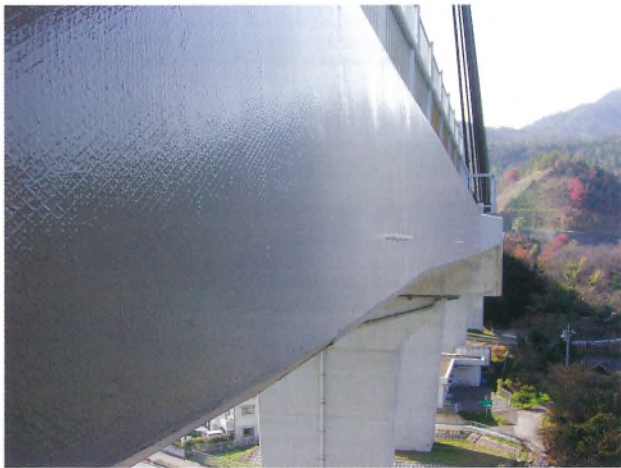
写真-7 コンクリート剥落防止工完了 Photo 7 Completed countermeasure against peel off of concrete
