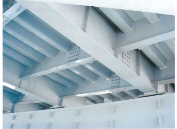
写真-6 塗替塗装後 (北備讃瀬戸大橋) Photo 6 After re-painting (Kita Bisan-Seto Bridge)
