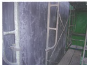
写真-7 下地処理完了（この後、炭素繊維シート巻立てを施工） Photo.7 Completion of Base Treatment (after the treatment carbon fiber sheet lining is executed)
