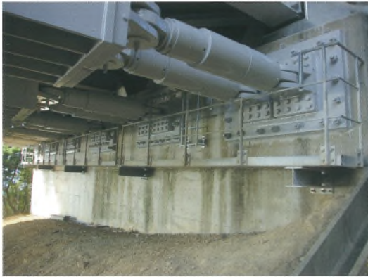
巻頭写真-29 上部工耐震補強 (ダンパー設置) Opening photo.29 Seismic upgrading for superstructure with damping devices ※ P 62 参照 (See page 62.)
