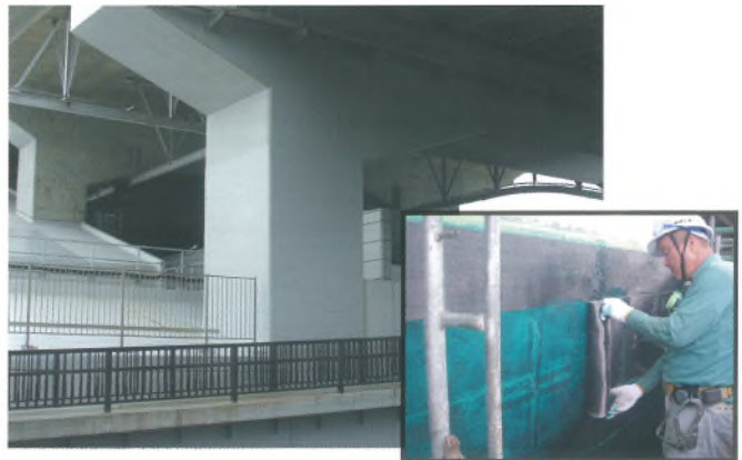
巻頭写真-34 橋脚の耐震補強 (炭素繊維巻立て) Opening photo.34 Seismic upgrading for piers (carbon fiber retrofitting method) ※ P 62 参照 (See page 62.)
