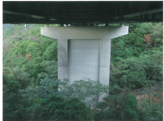
巻頭写真-39 6P橋脚補強完了(耐震壁増厚) Opening photo.39 Seismic retrofitting of 6P (increasing thickness of seismic resisting wall) ※ P 62 参照 (See page 62.)
