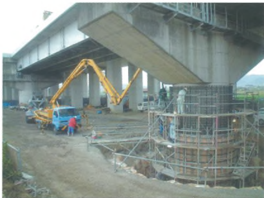
巻頭写真-33 橋脚の耐震補強 (RC 巻立て) Opening photo.33 Seismic upgrading for piers (reinforced concrete jacketing method)
