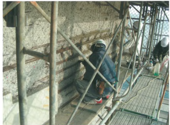
写真-41 剥落対策状況(防錆材塗布) Opening photo.41 Preventive work against scaling off ※ P 7、47 参照 (See page 7, 47.)
