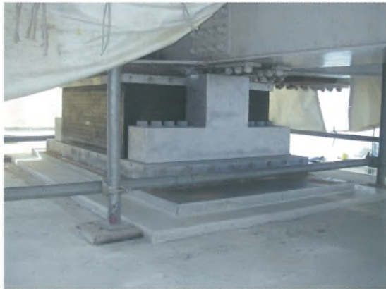
巻頭写真-31 免震支承への交換 Opening photo.31 Replacement to seismic isolation bearing ※ P 62 参照 (See page 62.)
