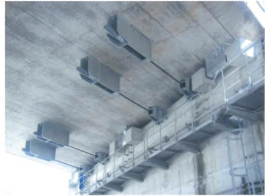
巻頭写真-30 落橋防止装置の設置 Opening photo.30 Seismic upgrading with unseating prevention system
