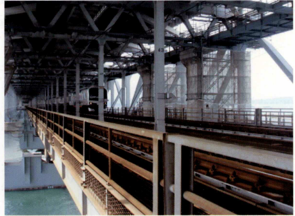
巻頭写真-9 北備讃瀬戸大橋補剛桁塗替 Opening Photo 9 Recoating of the stiffening girder in Kita Bisan-Seto Bridge
