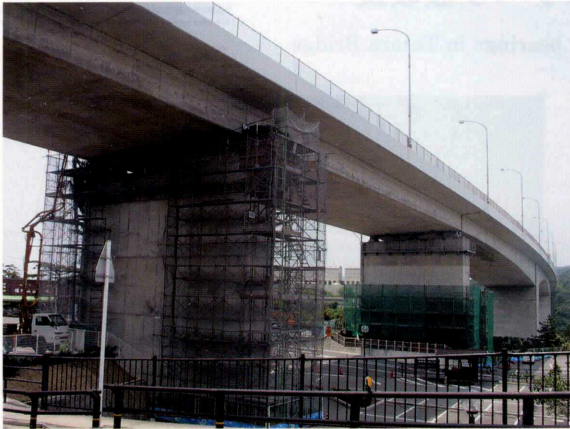
巻頭写真-8 2P, 3P施工状況 Opening Photo 8 Retrofitting work for 2P and 3P
