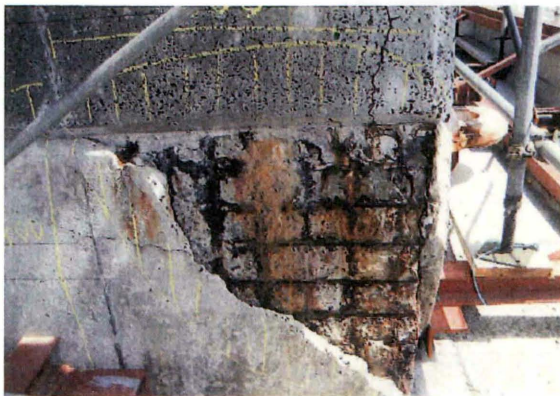
写真-3 基部の剥離・鉄筋露出 Photo 3 Steel bars at the base of the pier after chipping
