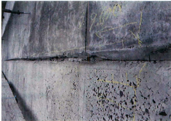
写真-2 目地の浮き Photo 2 Concrete floating at joint
