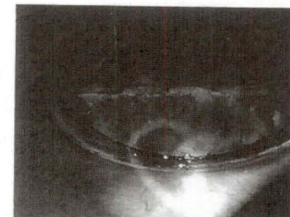
写真-2 滞水状況 Photo 2 Undrained condition
