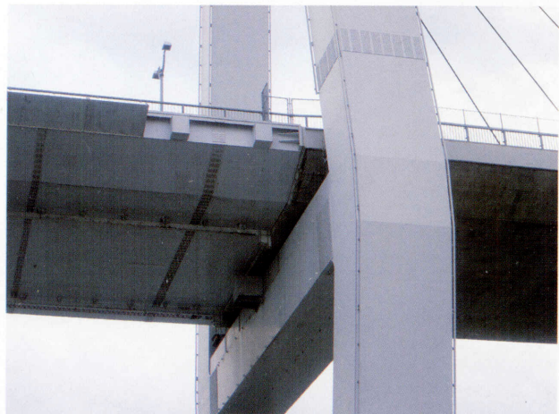
巻頭写真-12 生口橋 桁複合部 Opening Photo 12 Composite girder of Ikuchi Bridge
