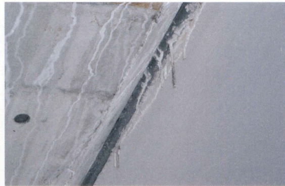
写真-9 接合部桁下の遊離石灰 Photo 9 Isolated lime at connections
