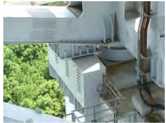
写真-10 段差防止工全景 Photo.7 Whole view of Prevention work for faulting of BVa2P
