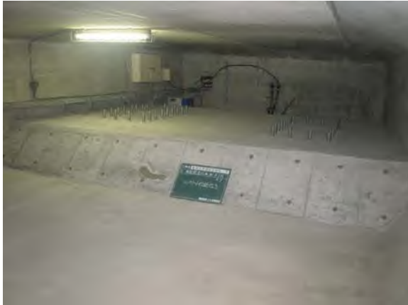
写真-4 箱桁内面の桁増し厚状況 (1A) Photo 4 Inside of thickened box girder (1A)
