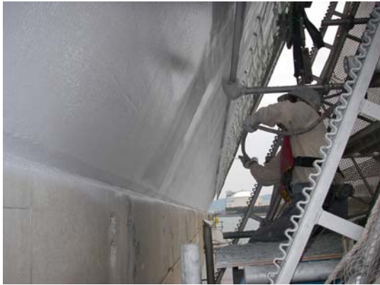
写真-6 南備讃瀬戸大橋7A南面中塗1層目施工状況 Painting (First middle coat) at 7A anchorage
