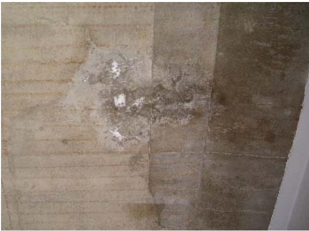
写真-2 因島大橋東高架橋 床板裏面状況 Photo.2 Underside of the deck (Innoshima-higasi Viaduct)
