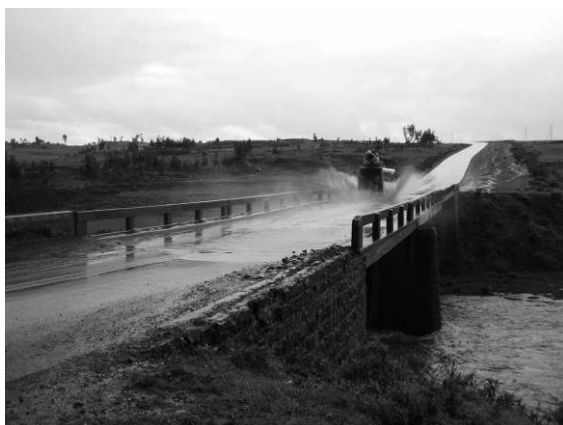
写真-7 雨季に滞水する橋 Photo 7 Water Ponding in Rainy Season
