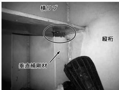
写真-1 縦桁と横リブの交差部 Phot.1 Connection of stringer and lateral rib
