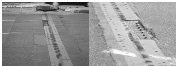
写真-2 伸縮装置の管理状態 Photo 2 Maintenance Condition of Expansion Joint
