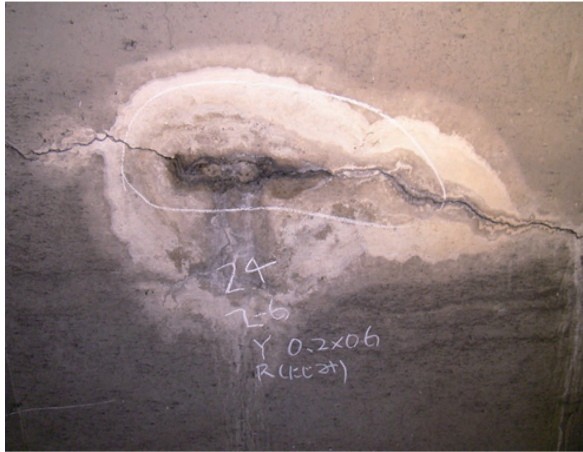
写真-4 遊離石灰析出箇所 Photo.4 Deposit of free lime
