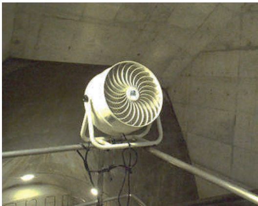
写真-1 SB1A送風機設置状況 Photo.1 situation of blower system (SB1A)
