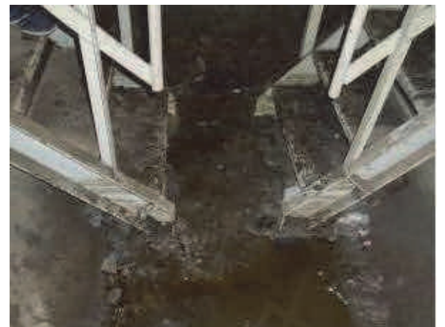
写真-9 アンカレイジ内滞水 Photo 9 Undrained Water in Anchorage
