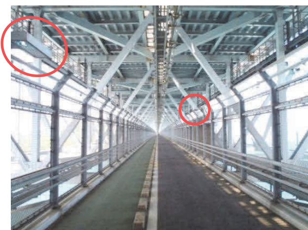
写真-1 配置状況 Photo.1 Lightings for the bicycle and pedestrian way
