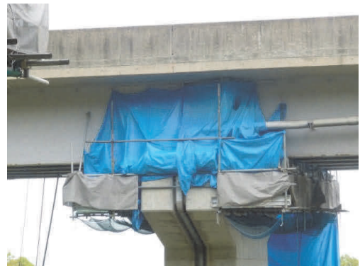
写真-5 施工箇所の粉じん飛散防止 Photo 5 Scatter prevention sheet around retrofitting work
