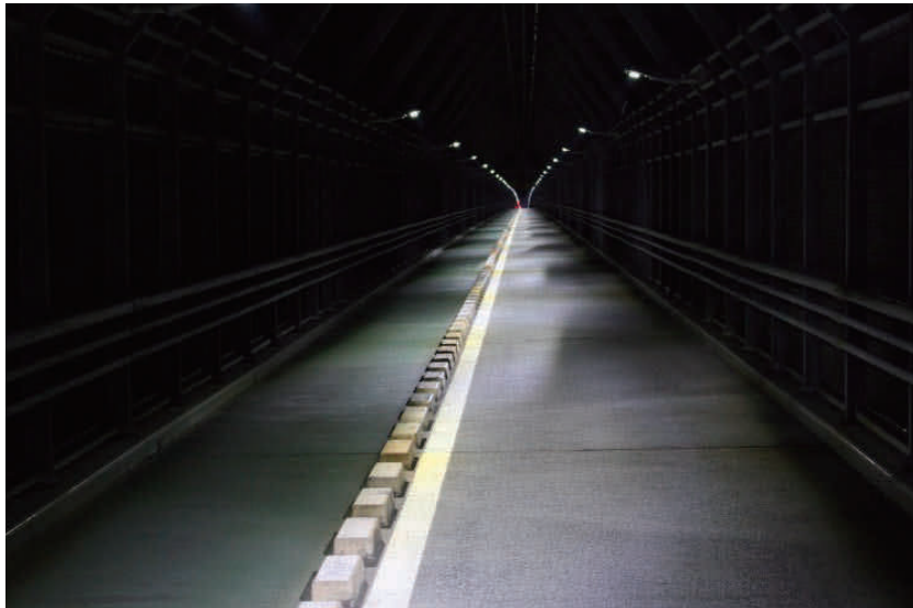
写真-9 LED 照明夜間点灯状況 LED lighting at night-time
