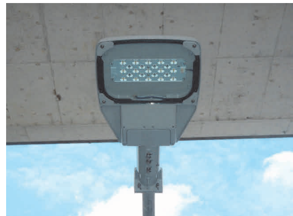
写真-4 LED 照明器具
