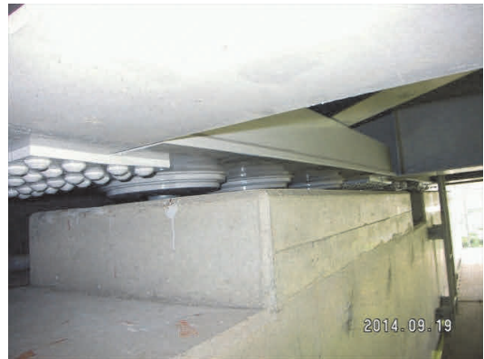
写真-12 縦型緩衝ピン+横梁の設置 Photo 12 Vertical buffer anchor pin and additional beam at girder end
