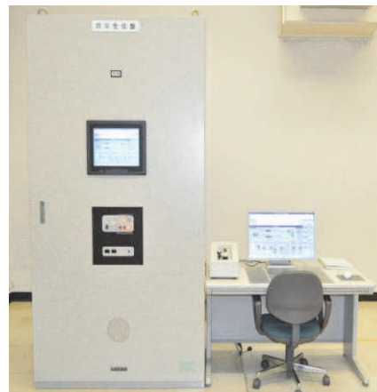
写真-2 新防災受信盤 Photo 2 New Disaster prevention reception board
