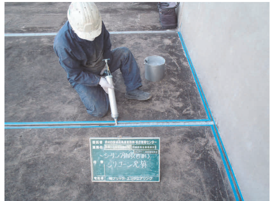
図-11 PCパネル目地の補修 Fig.11 Repair of the joint of the pre-cast concrete
