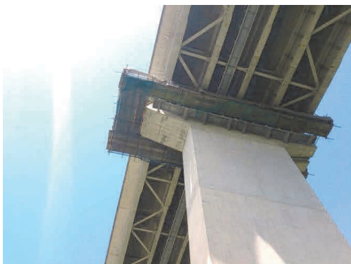
写真-4 橋脚天端周囲に設けた足場 Photo 4 Suspended scaffolding around the pier cap
