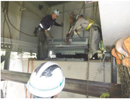
写真-8 狭あいな施工箇所での部材設置 Photo 8 Installation of retrofitting member in narrow space
