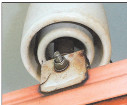
写真-5 絶縁碍子内部の汚損 Photo 5 Contaminated insulator
