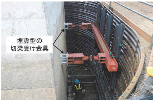
写真-8 埋設型の切梁受け金具設置状況 Photo 8 Attachment for short strut (buried type)
