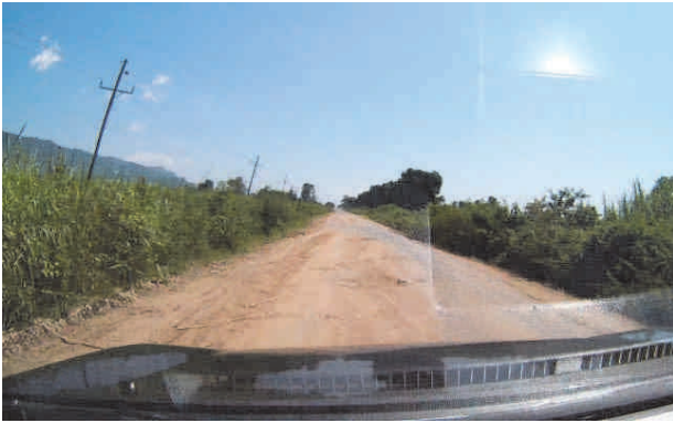
写真-1 状態の悪い舗装道路の例 Photo 1 An example of paved road in not good condition
