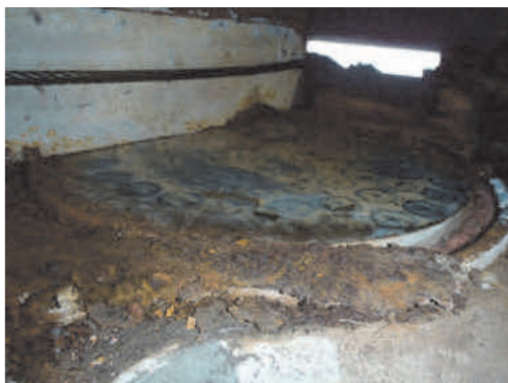
写真-3 上沓下沓間のさび等の状況 Photo 3 Corrosion between top and bottom bearing
