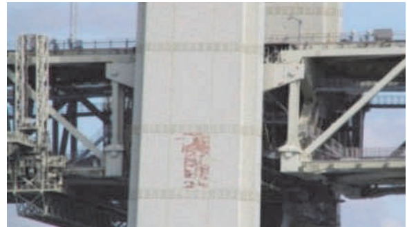
写真-2 明石海峡大橋主塔の塗膜剥離 Photo 2 Coating peeling at main tower of Akashi Kaikyo Bridge
