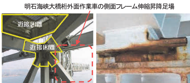
写真-9 近接困難箇所と鋼床版縦桁支承部局部腐食状況 Photo 9 Hard-to-reach area and localized corrosions
