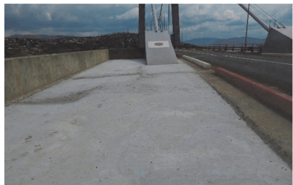
写真-8 防水工の状況(2A上流側) Photo 8 Status of waterproofing workers (2A upstream side)
