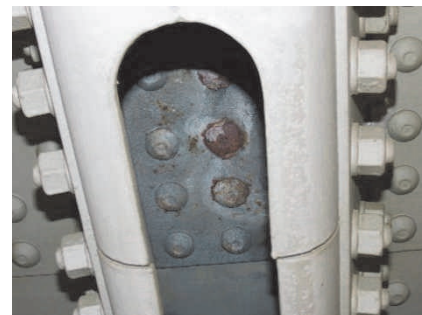
写真-4 鋼床版添接ボルトの腐食 Photo 4 Corrosion of steel slab injection bolt
