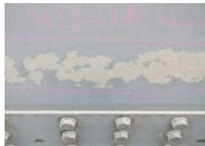
写真-3 来島海峡第二大橋の塗膜剥離 Photo 3 Coating peeling at girder of 2nd Kurushima Kaikyo Bridge
