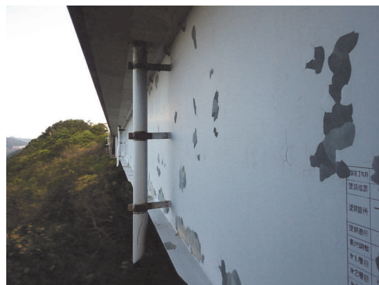
写真-2 はがれ(主桁外面ウェブ面) Photo 2 Peeling on the web of main girder
