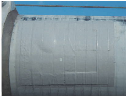
写真-2 補修テープの膨れ Photo 2 Expansion of a repair tape
