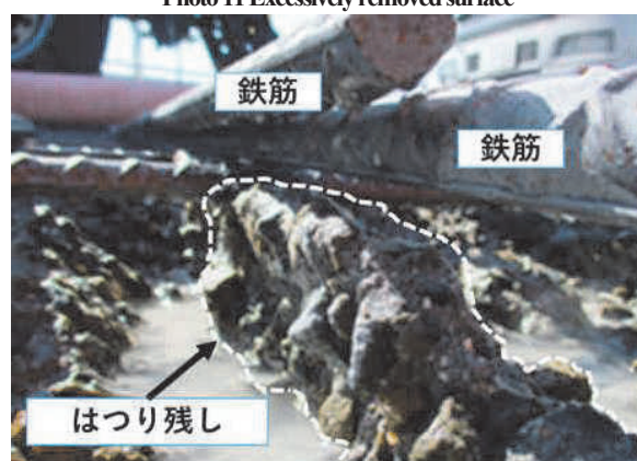
写真-12 鉄筋下のはつり残し Photo 12 Remained concrete portion under reinforce bars
