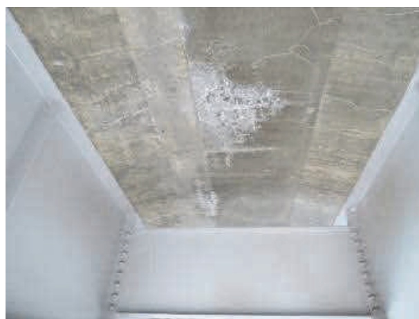
写真-4 床版下面の遊離石灰 Photo 4 Free lime of lower surface of the slab
