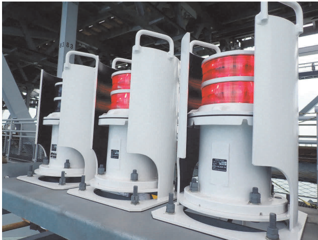
写真-4 LED 橋梁灯近接写真（南備讃瀬戸大橋R二灯） Photo 4 Closeup of LED bridge light (Minami Bisan-Seto Bridge R2)
