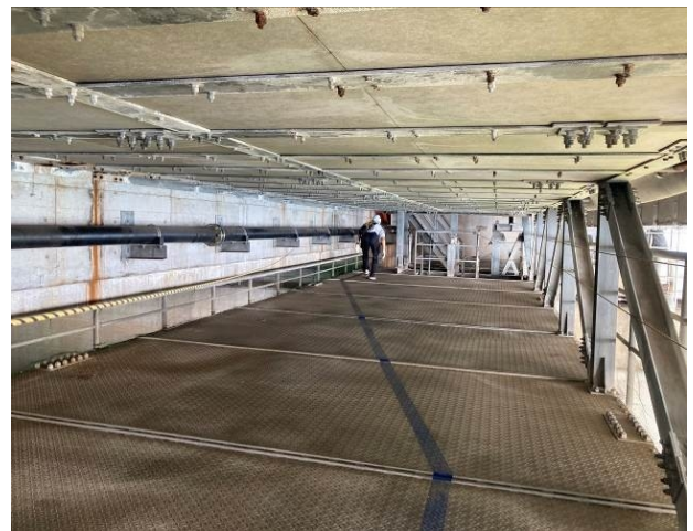
Low Overhead Clearance Narrow Walkway
